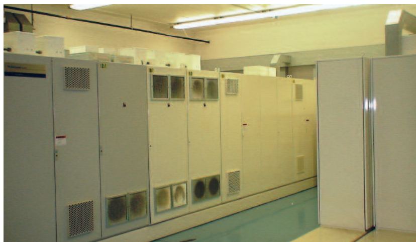
POWER IS FILTERED AT THE DRIVE CABINETS BECAUSE OF THE AMOUNT OF SENSITIVE EQUIPMENT IN A HIGH VOLUME ACTION AREA.
